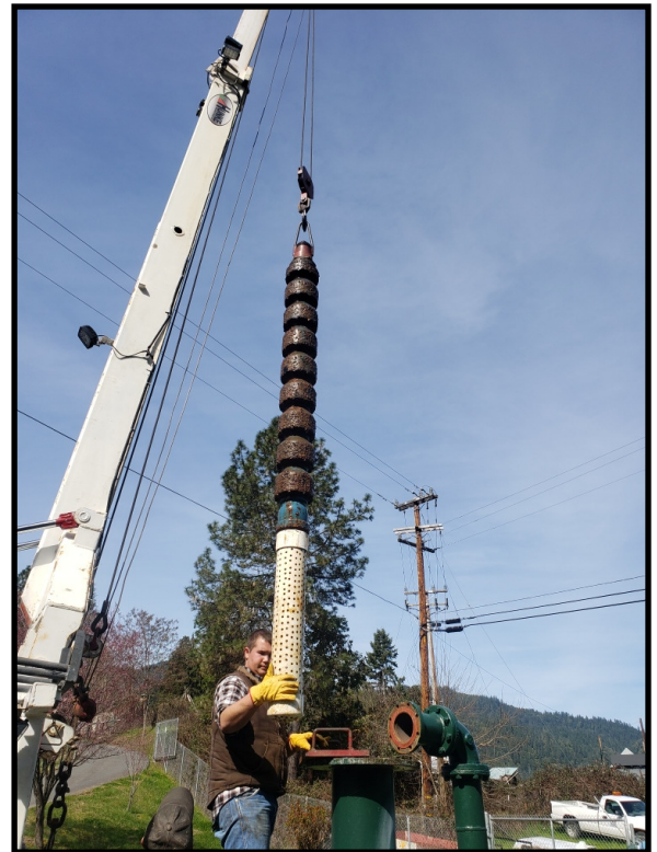
Removing old Pump #3 at the Albert E. Hodgson Water Treatment Plant. The pump was replaced in the Spring of 2019.
